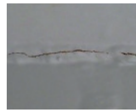
Fissuration de la protection anticorrosion
